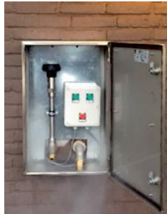
Remote filling box
